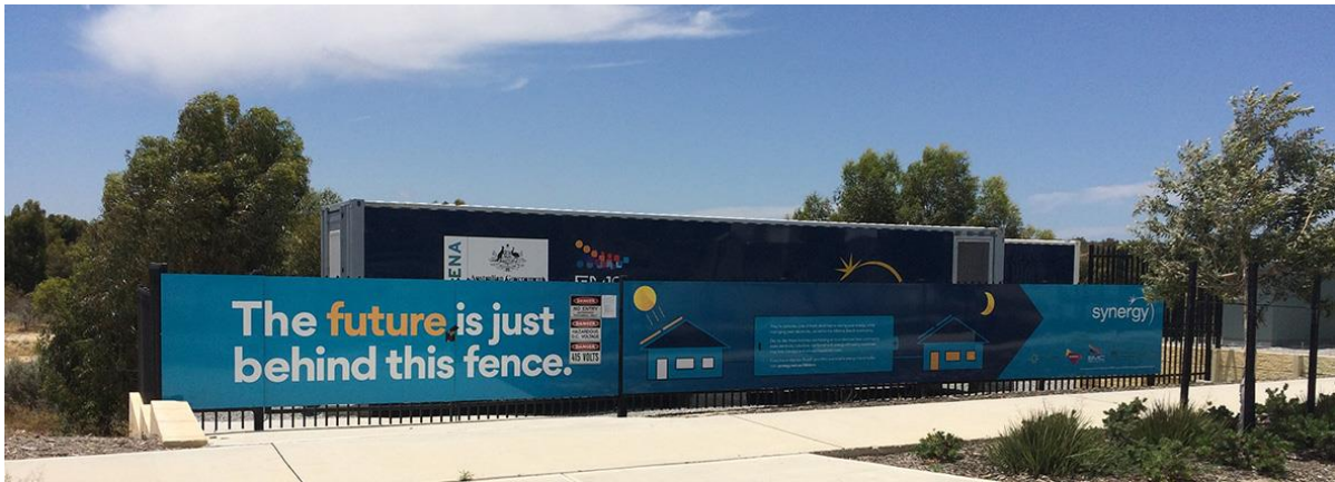
Figure 2.3: The site of the first community battery storage trial in Alkimos Beach.
